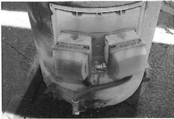
Item 2 - Pole Base Outlets
